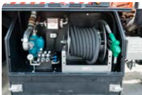
Fuel Pump and Hose Reel
